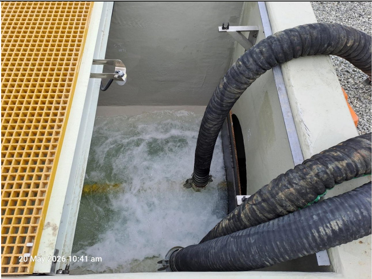
Photo – STP Inlet Works
