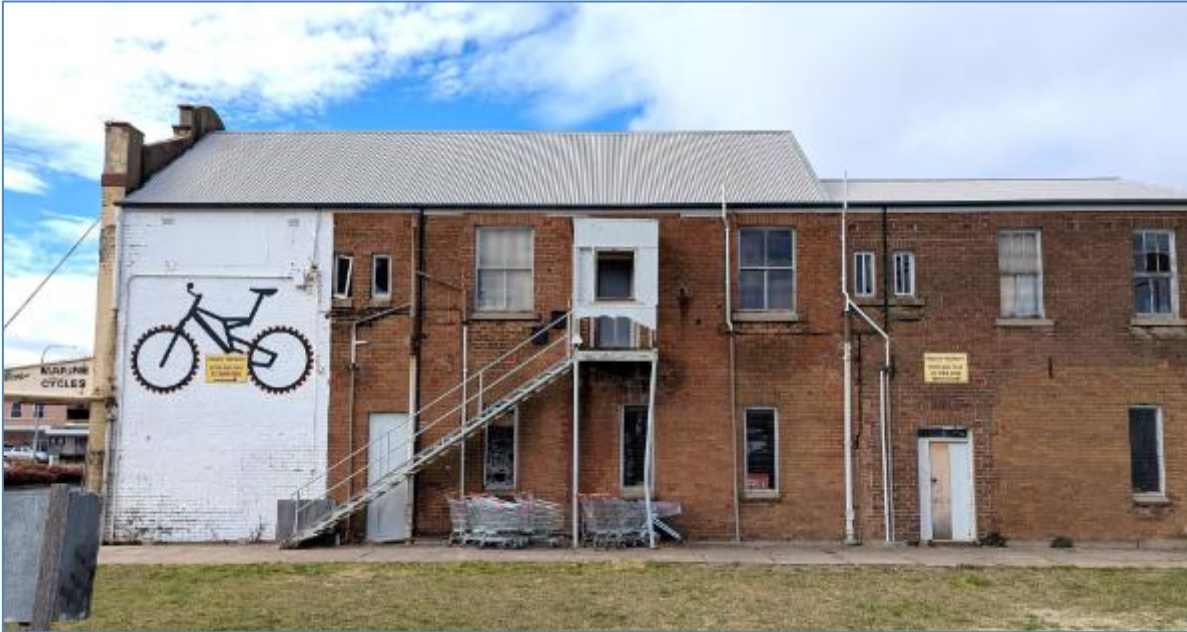
Figure 33 – view to the west facing elevation showing changes to the building in brickwork
