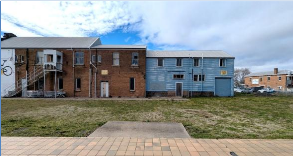
Figure 34 – view to the timber rear section of west facing elevation - building interior
