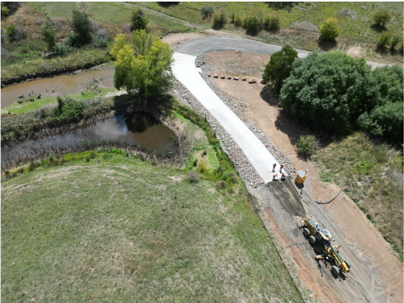
Photo – Lone Pine – Completion of the road works tie ins for either end of the culvert.
