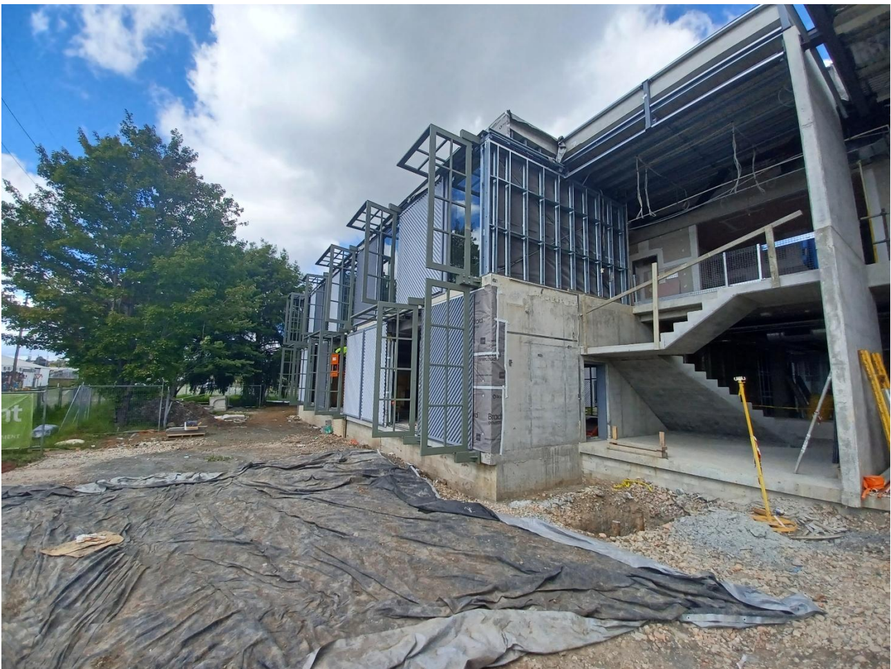
Photo – Construction of Orange Conservatorium and Planetarium – External view of the March St side of the building
