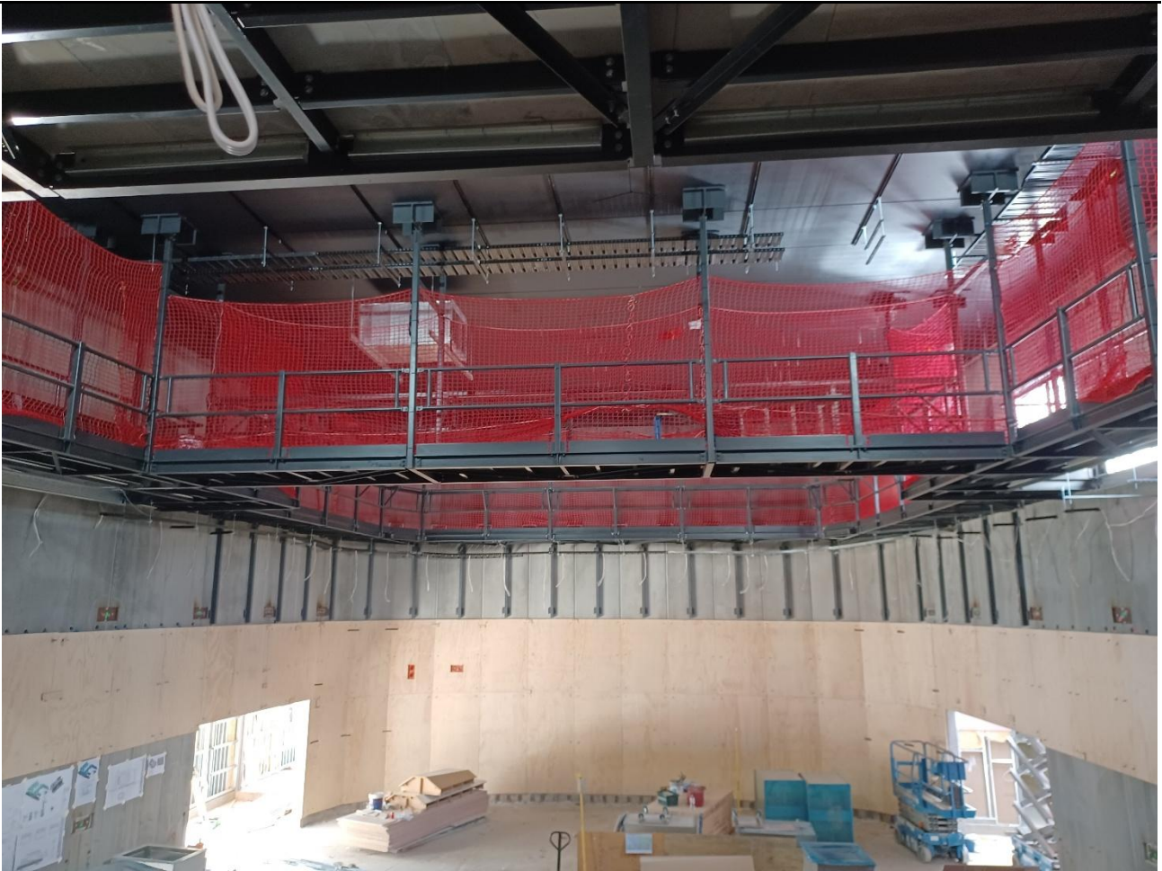
Photo – Construction of Orange Conservatorium and Planetarium – Internal view of the Recital Hall
