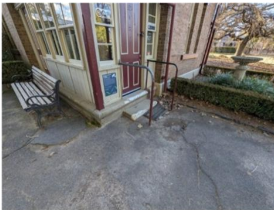
4. Close view. Note that there is damage to the perimeter bull nose edge on the original verandah which should be repaired and form part of the works.
