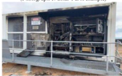
(Photograph 2: Fire damaged Inverter post fire event)
