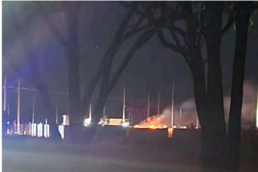
Crews worked throughout the night to contain the blaze. (Supplied: David Bailey)
