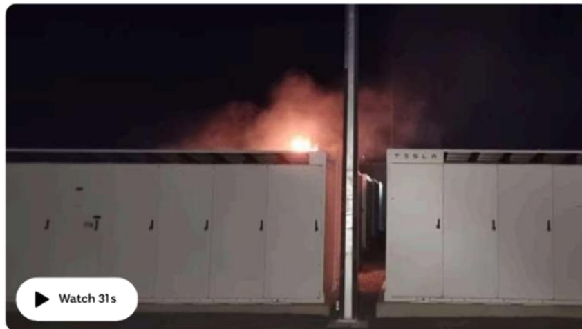
Fire breaks out at Tesla battery facility in Central Queensland. (Supplied: Kent Murray)
