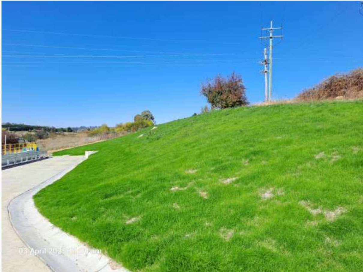
Photo: Establishment of grass on batters and tidy up works ongoing at STP
