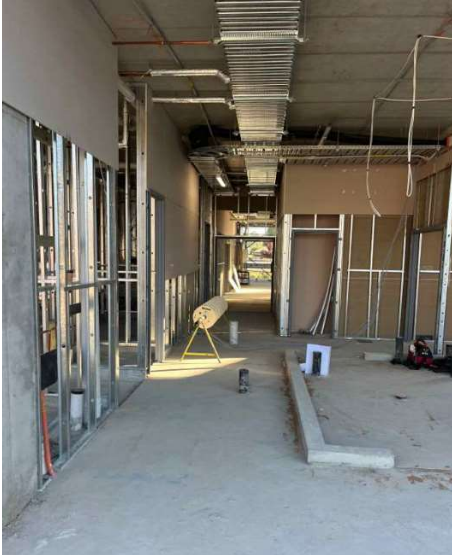
Photo – Construction of Orange Conservatorium and Planetarium internal view of the Recital Hall
