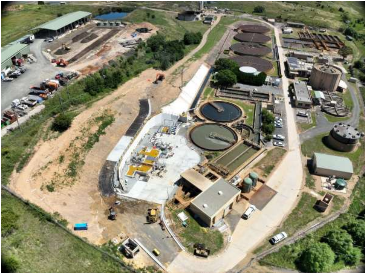
Photo: Site Photo of STP, new works shown lower left of centre
