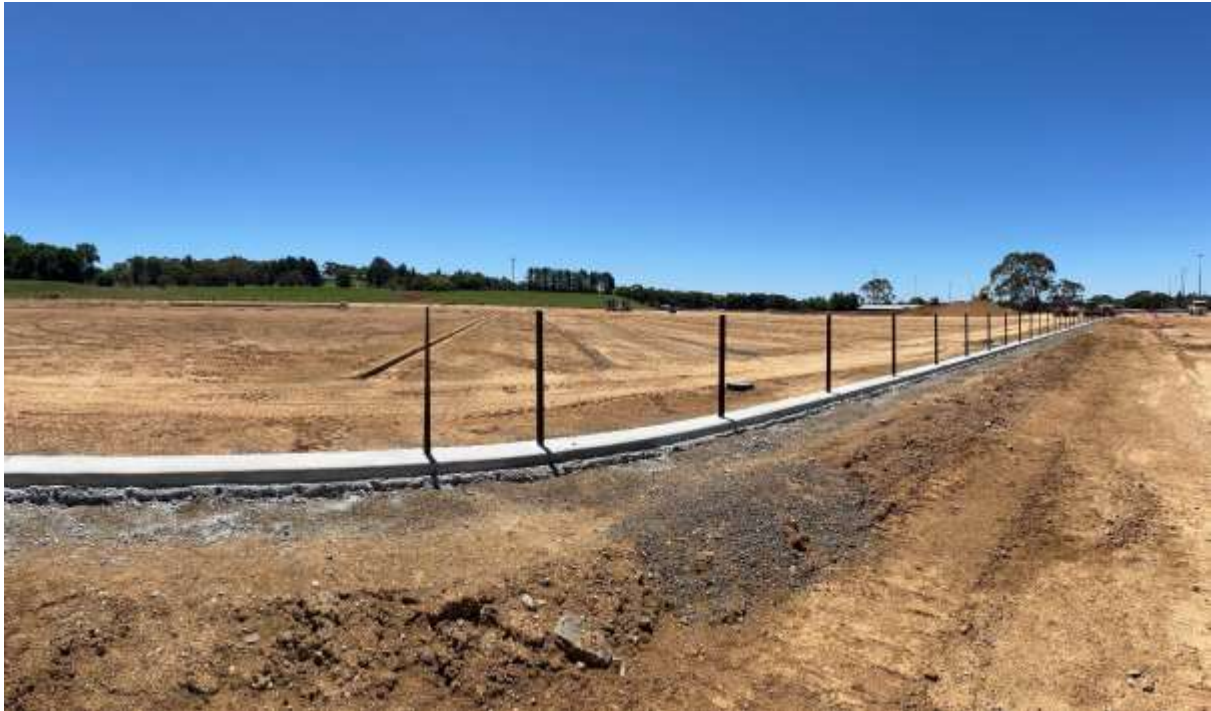
Photo – Installation of fencing and kerbing around the perimeter of the field.
