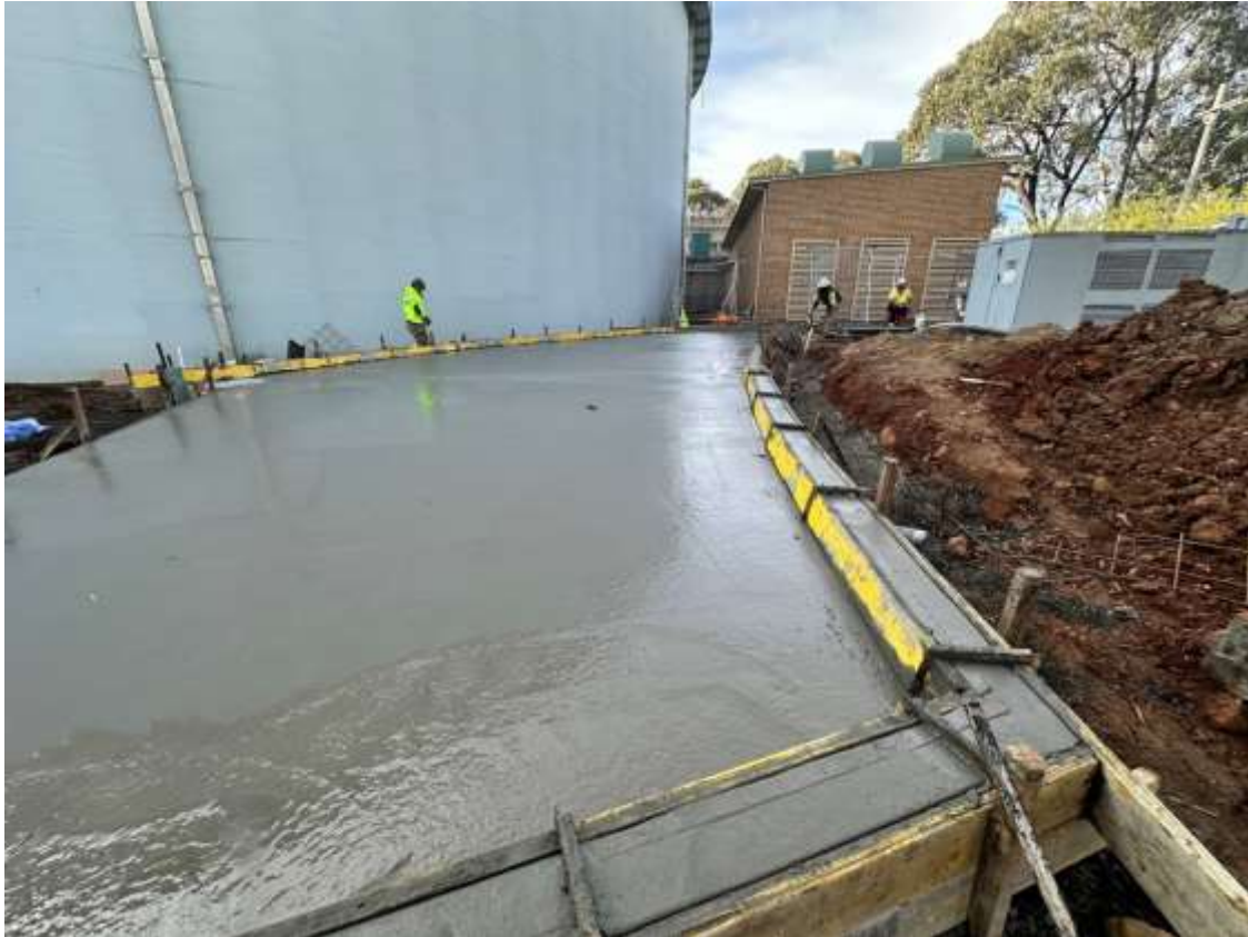
Photo – Icely Road WTP
