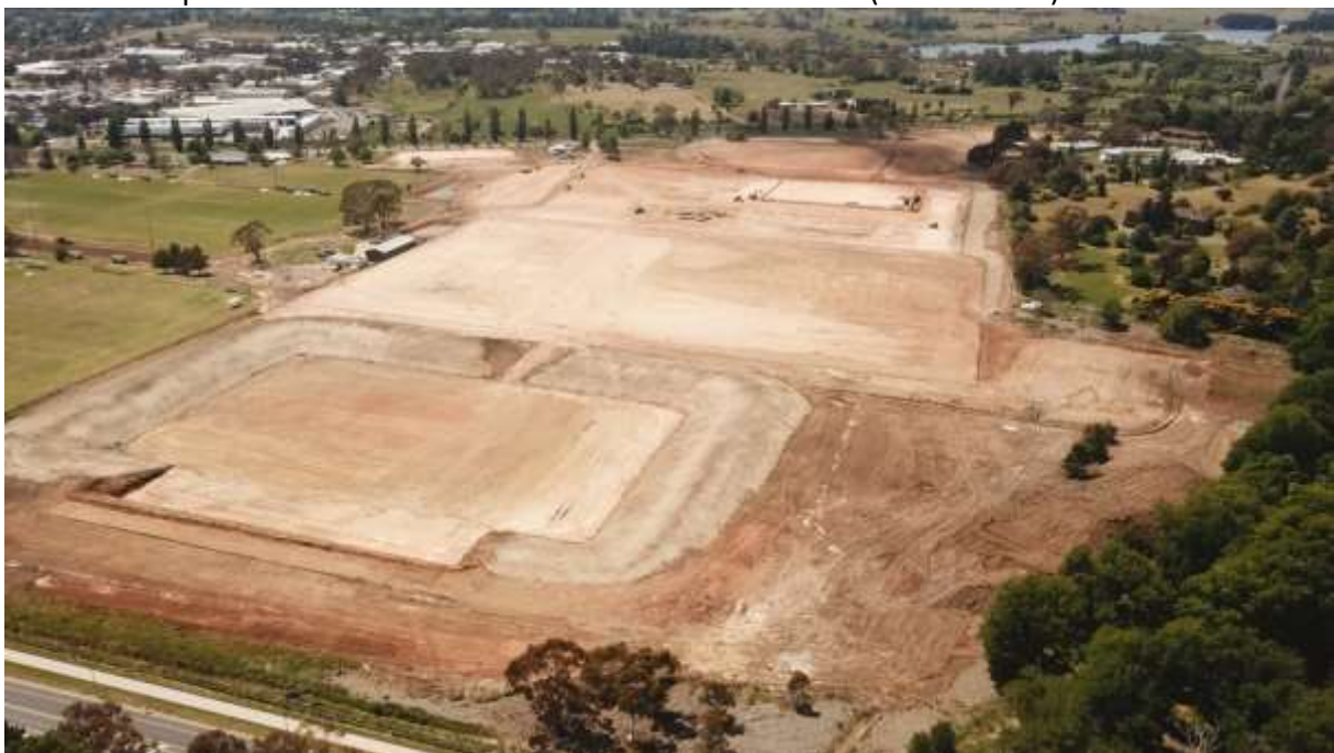
View of completed earth works from Main Stadium Precinct (Forest Road) side
