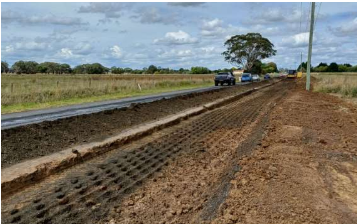
Photo: Excavation of unsuitable base materials in pavement widening area - Forest Road
