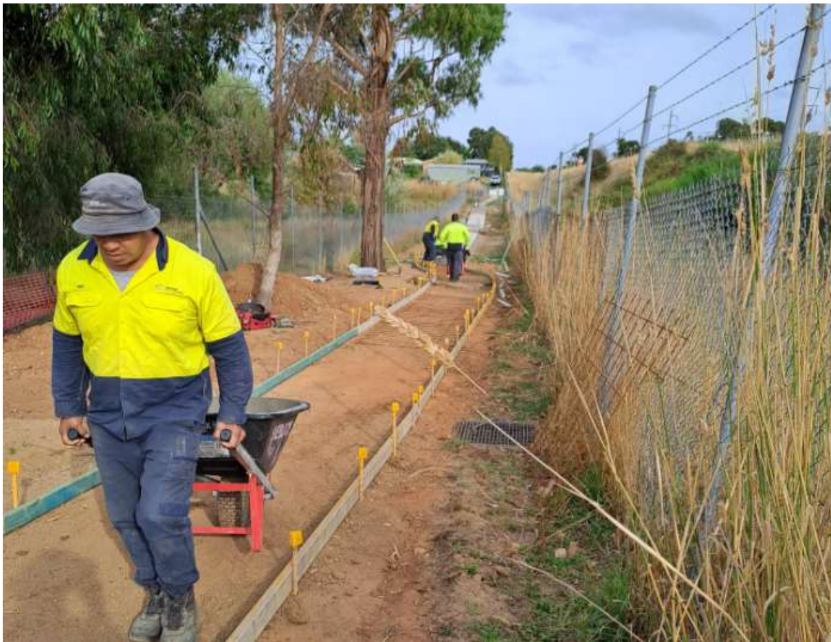
Photo: Crews wheelbarrowing concrete to the path for the Christian School due to access difficulties
