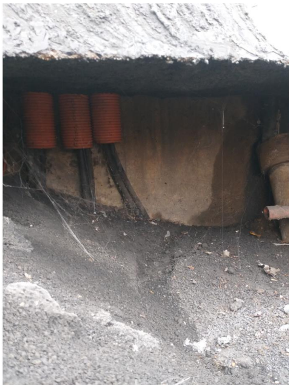
Photo – 500mm void found under carpark concrete slab (Woolworths building services in background)
